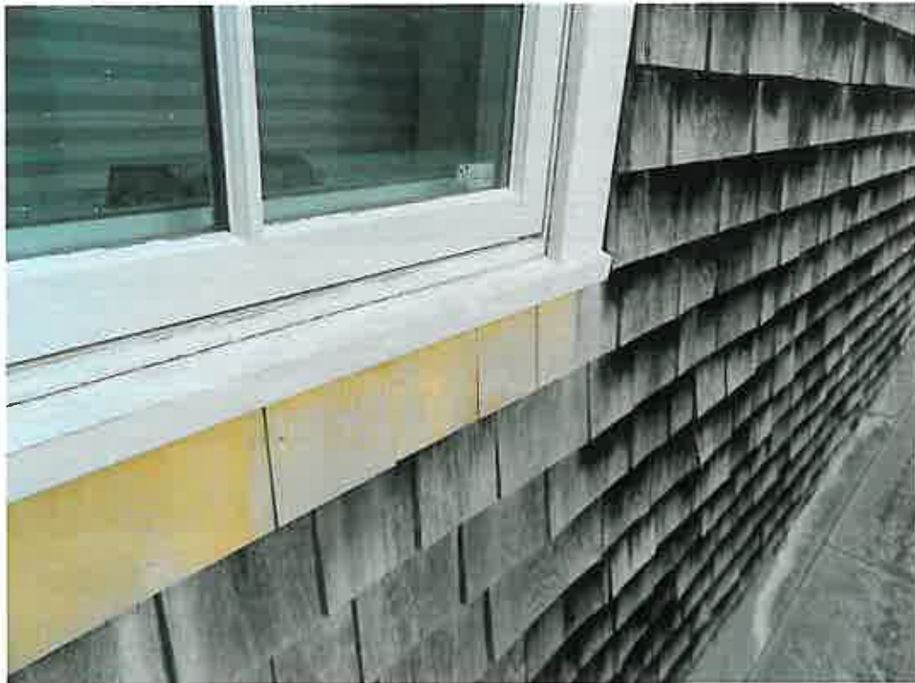
STAINLESS STEEL FACE NAILS ON RECENTLY REPLACED SHINGLES
