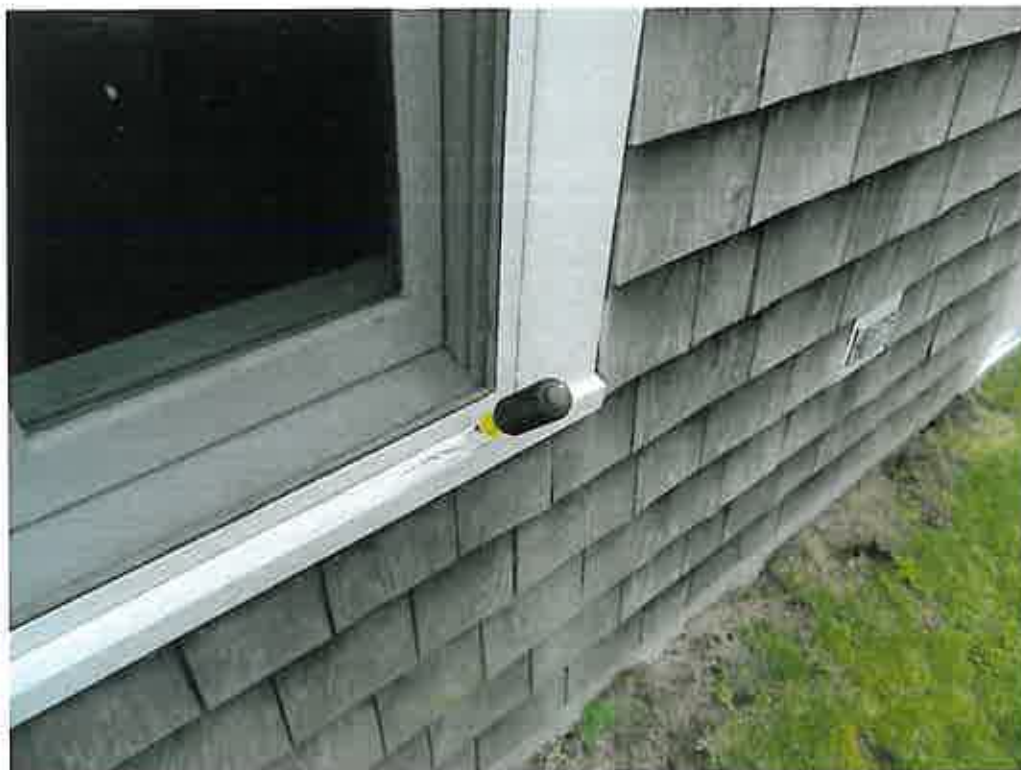
SEVERELY DETERIORATED WINDOW SILL LIKELY AFFECTING THE BUILDING ENVELOPE
