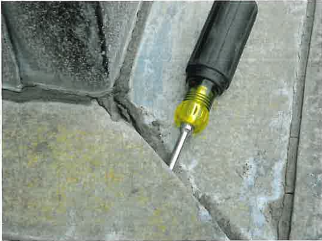
FAILED SEALANT AT THE LCC LOW-SLOPED ROOF
