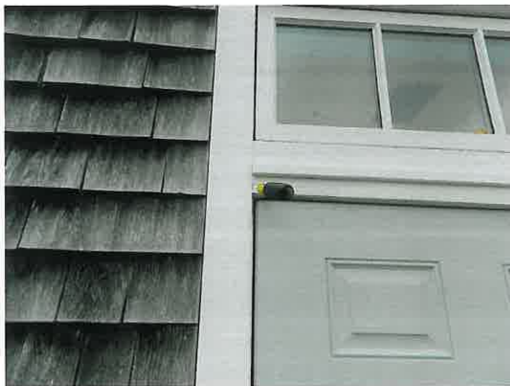
SEVERELY DETERIORATED DOOR FRAME
