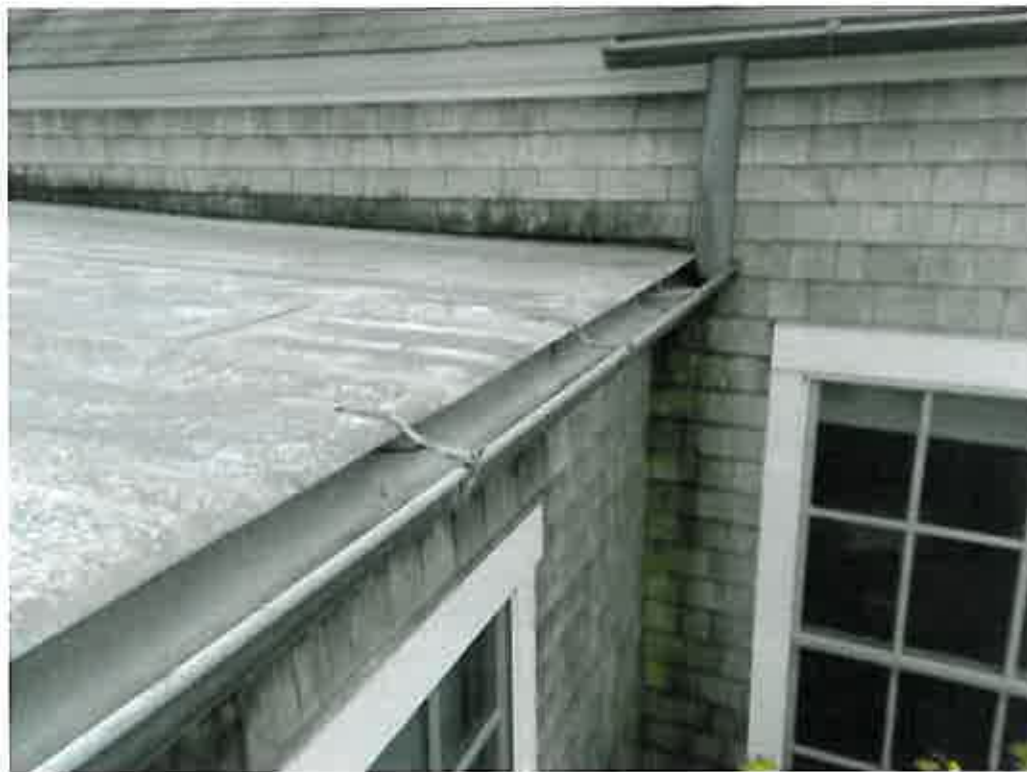
OVERVIEW OF A TYPICAL GUTTER CONFIGURATION AT THE CHILMARK SCHOOL, NOTE- DOWNSPOUTS BEING DIRECTED INTO A LOWER GUTTER OF INSUFFICIENT SIZE TO CARY THE RUNOFF
