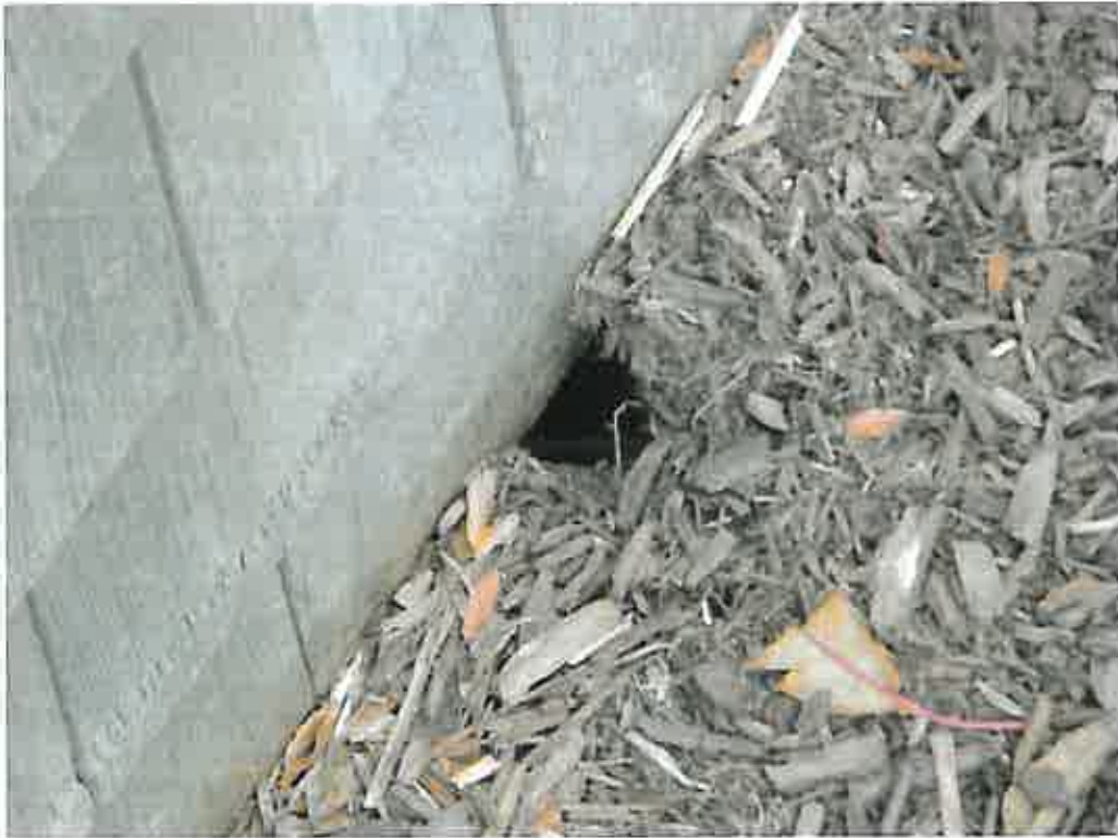
RODENT HOLE AT LOCATION OF SIDING IN CONTACT WITH GRADE
