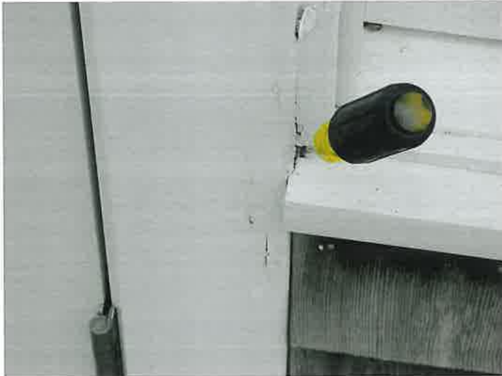
SEVERELY DETERIORATED WINDOW-TO-DOOR FRAME TRANSITION
