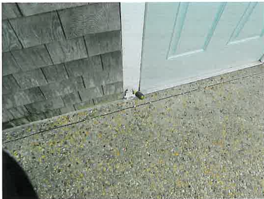
MORE DETERIORATED DOOR TRIM AND LIKELY DOOR FRAME DETERIORATION
