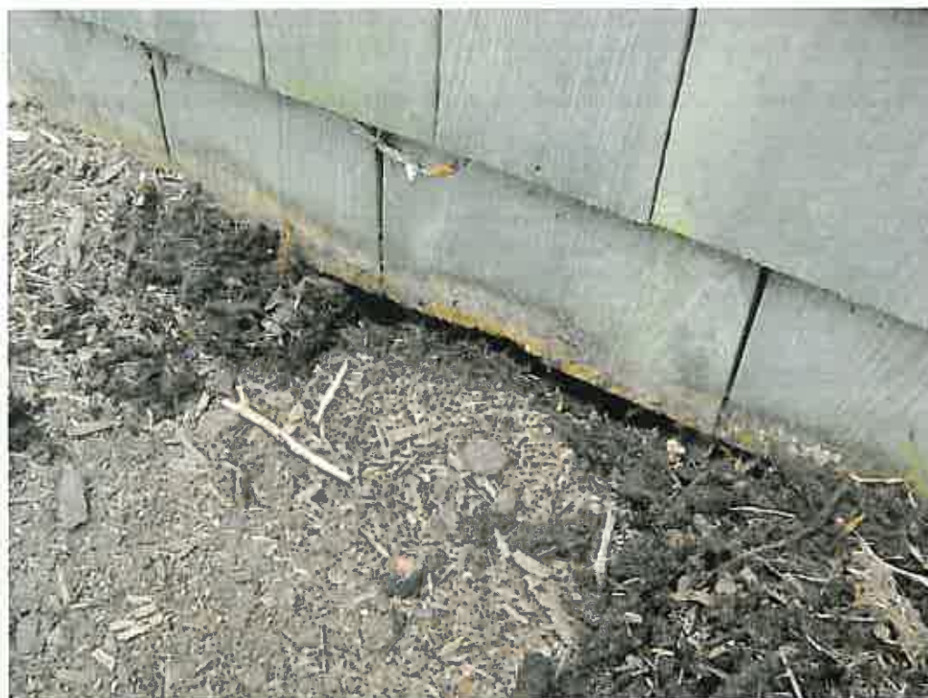
MORE DETERIORATED SIDING IN CONTACT WITH GRADE
