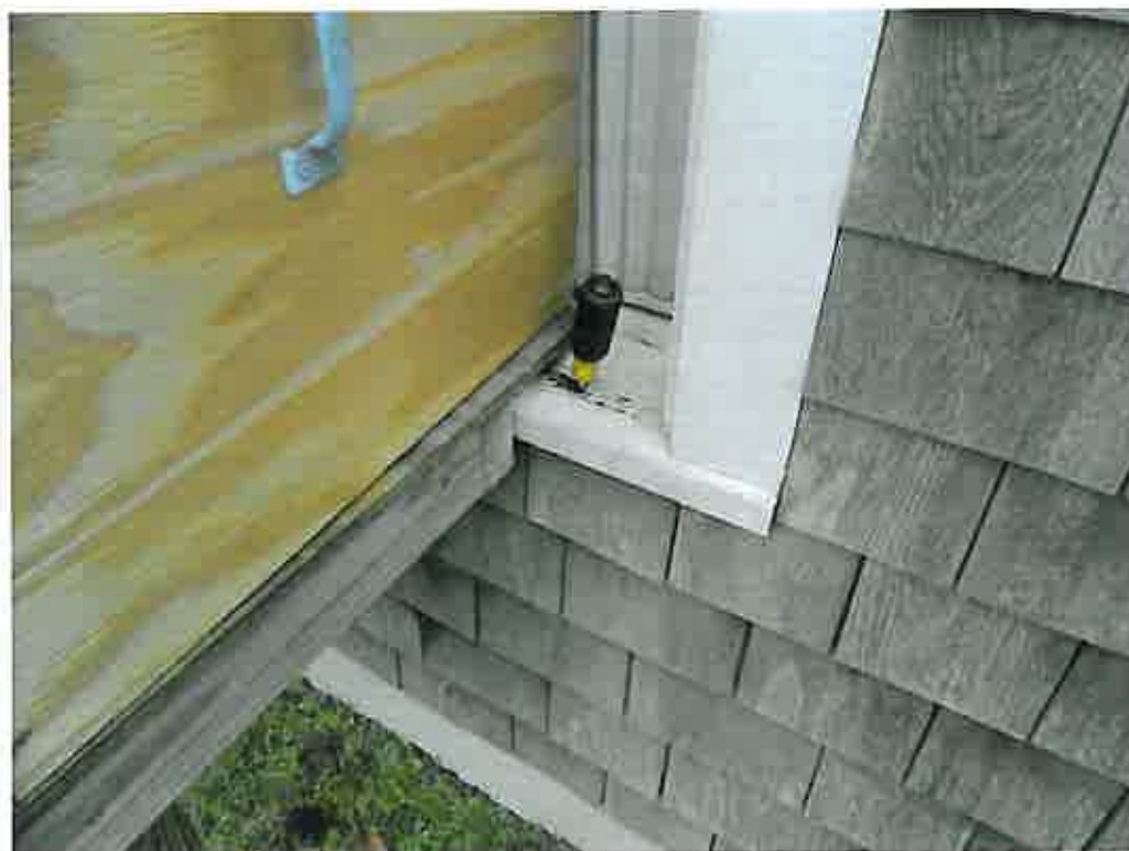
ANOTHER SEVERELY DETERIORATED WINDOW SILL
