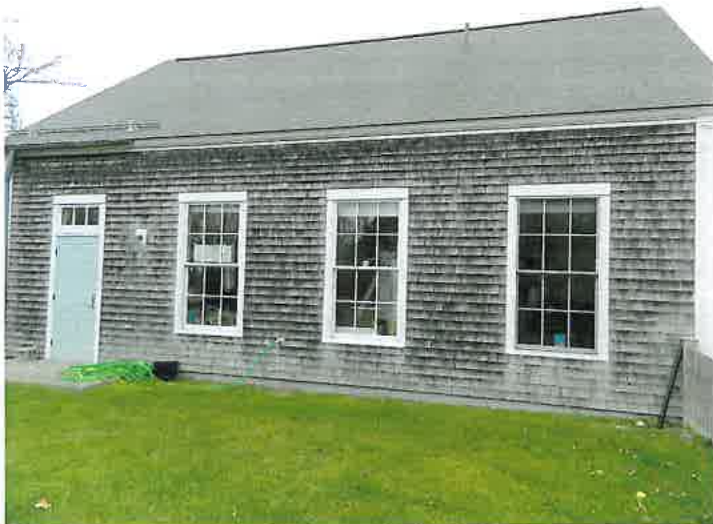
ROOF PLANE DIRECTING THE MAJORITY OF ITS RUNOFF DIRECTLY TO SURROUNDING GRADE
