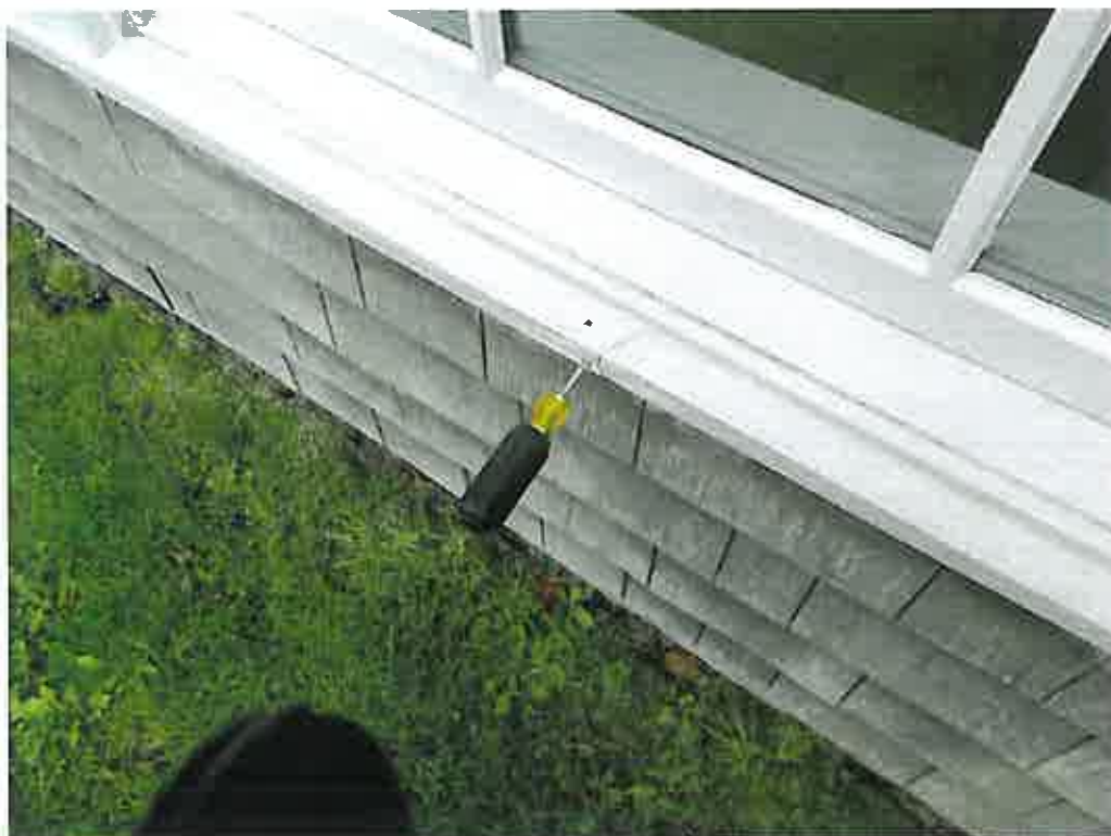
SEVERELY DETERIORATED WINDOW SILL AT COURTYARD LOCATION
