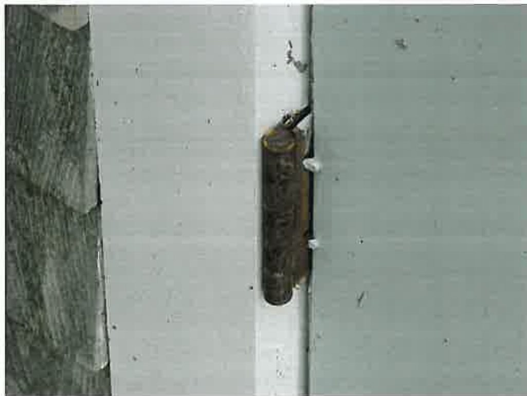
RUSTING DOOR HINGE, IMPROPER HARDWARE FOR THIS ENVIRONMENT
