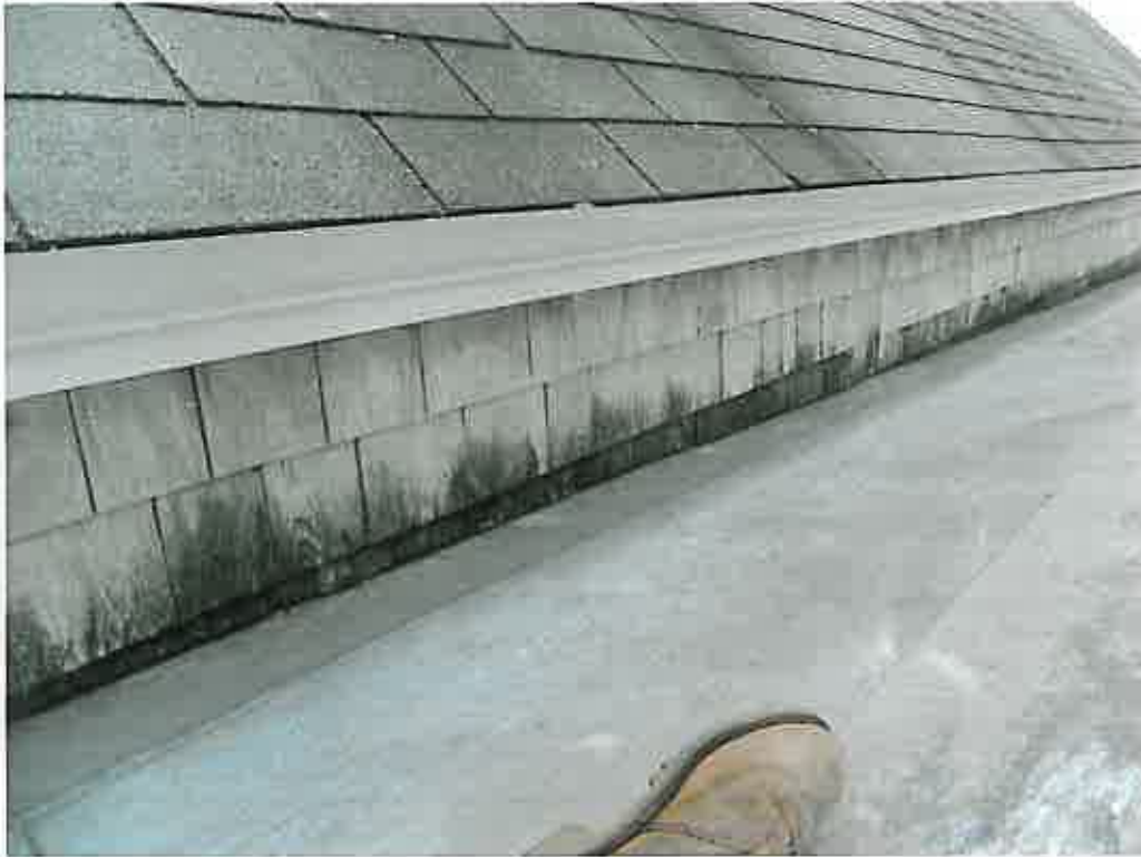
ROOF PLANE DIRECTING ROOF RUNOFF TO LOWER ROOF WHICH DRAINS TO THE GUTTER OF INSUFFICIENT SIZE DEPICTED ABOVE
