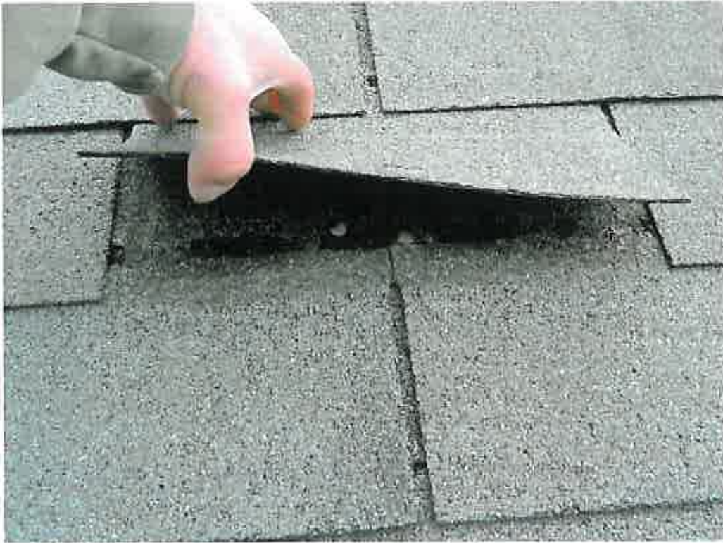
TYPICAL HIGH NAILING OF THE ASPHALT SHINGLES
