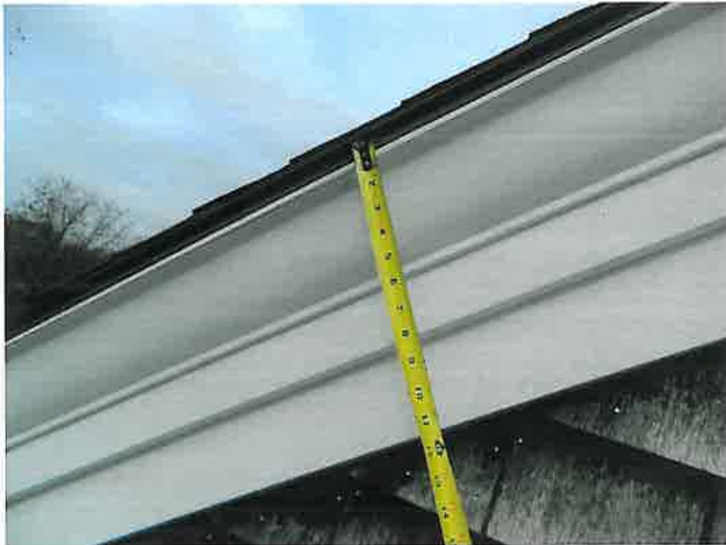
CEDAR RAKE TRIM IN VERY GOOD CONDITION
