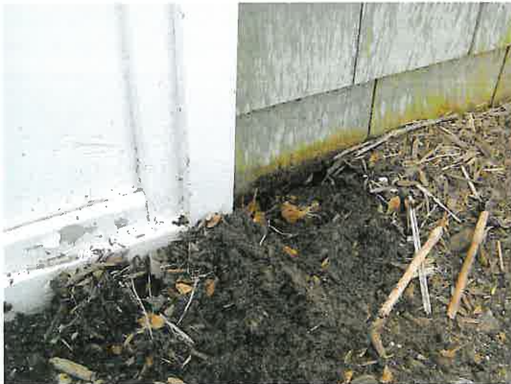
DETERIORATED SIDING IN CONTACT WITH GRADE
