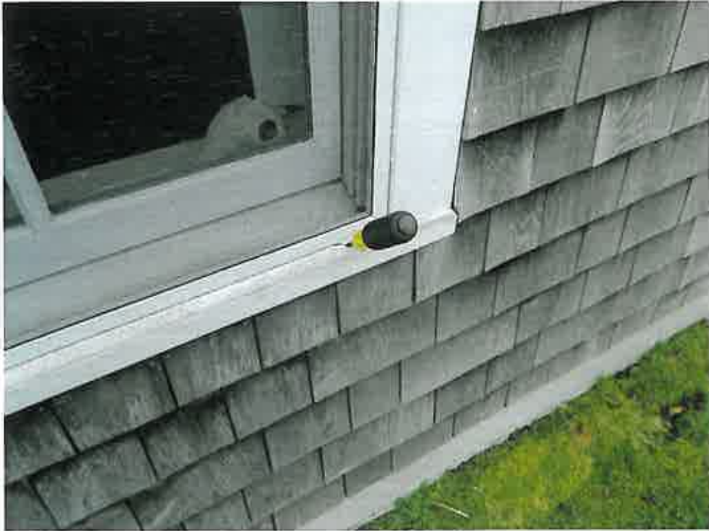
ANOTHER SEVERELY DETERIORATED WINDOW SILL
