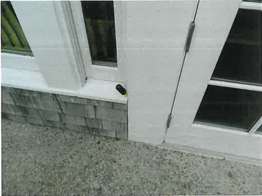
ANOTHER DETERIORATED WINDOW-TO-DOOR TRANSITION WITH LIKELY FRAMING DETERIORATION
