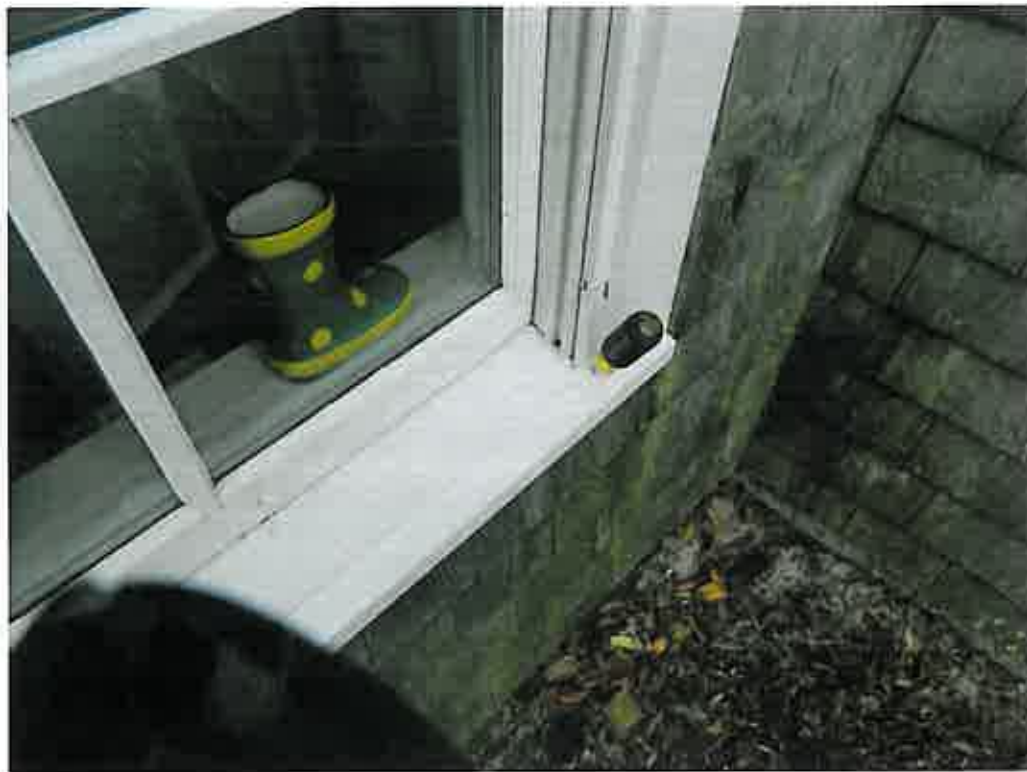
ANOTHER SEVERELY DETERIORATED WINDOW SILL
