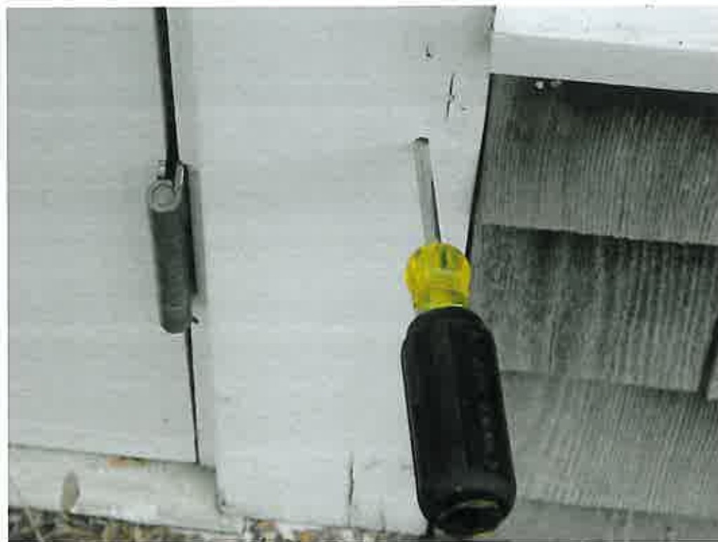
SEVERELY DETERIORATED DOOR TRIM
