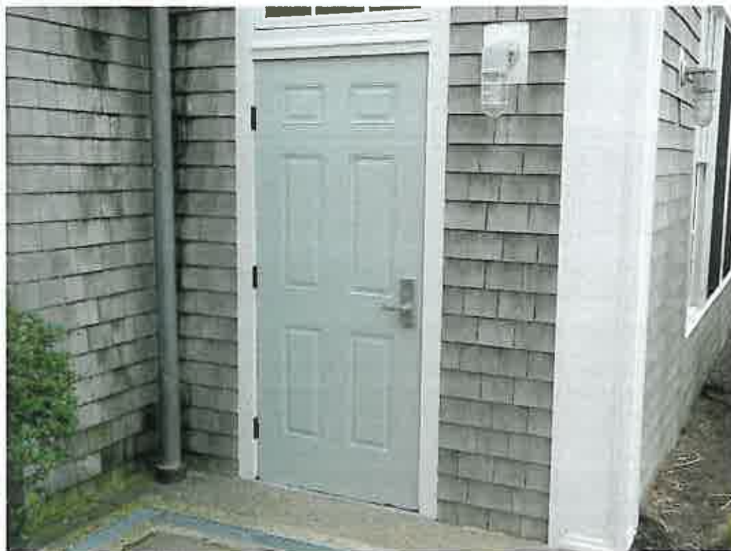
SIDING IN CONTACT WITH WALKWAY/GRADE
