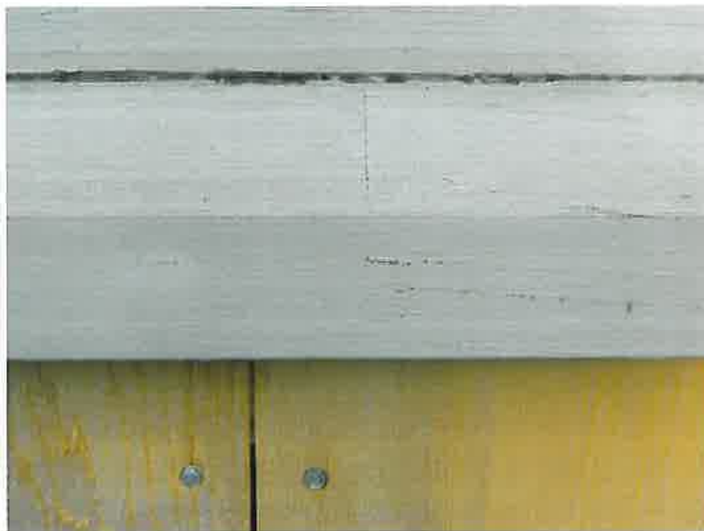
FINGER JOINTED PINE WINDOW SILL AND SASH SHOWING SIGNS OF THE EARLY STAGES OF FAILURE
