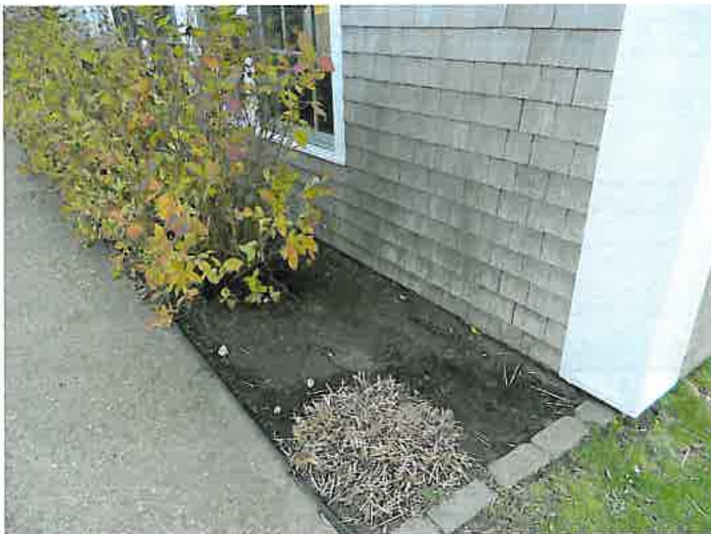
SIDING NEARLY IN CONTACT WITH GRADE, NOT CODE COMPLIANT
