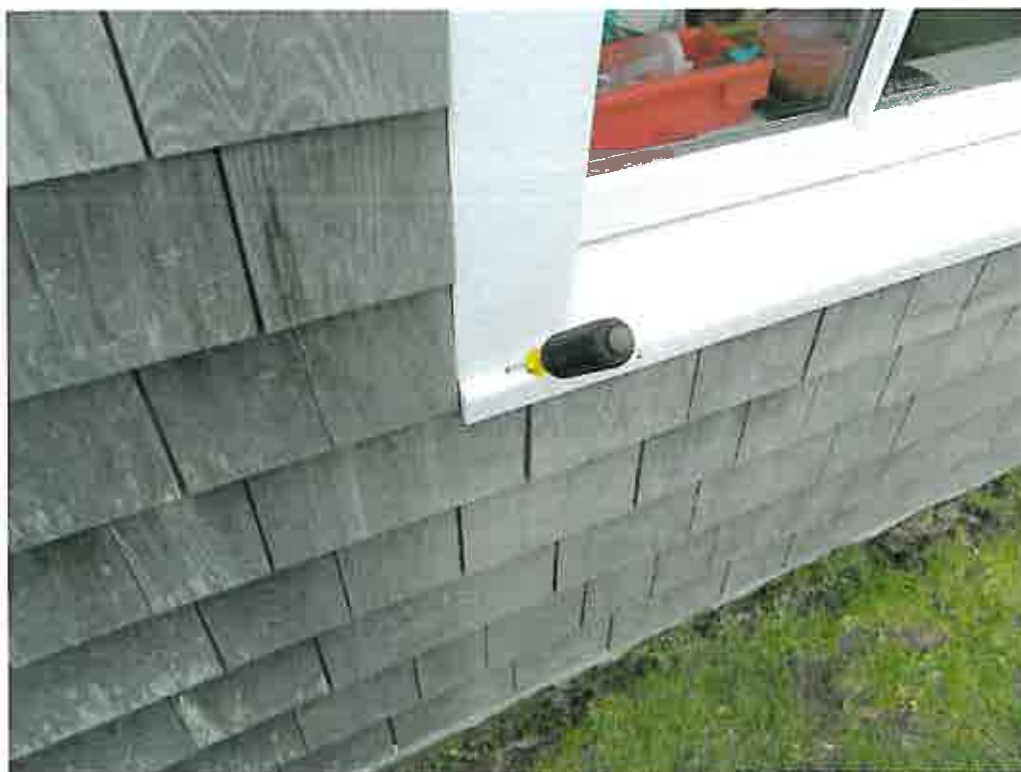
ANOTHER SEVERELY DETERIORATED WINDOW SILL
