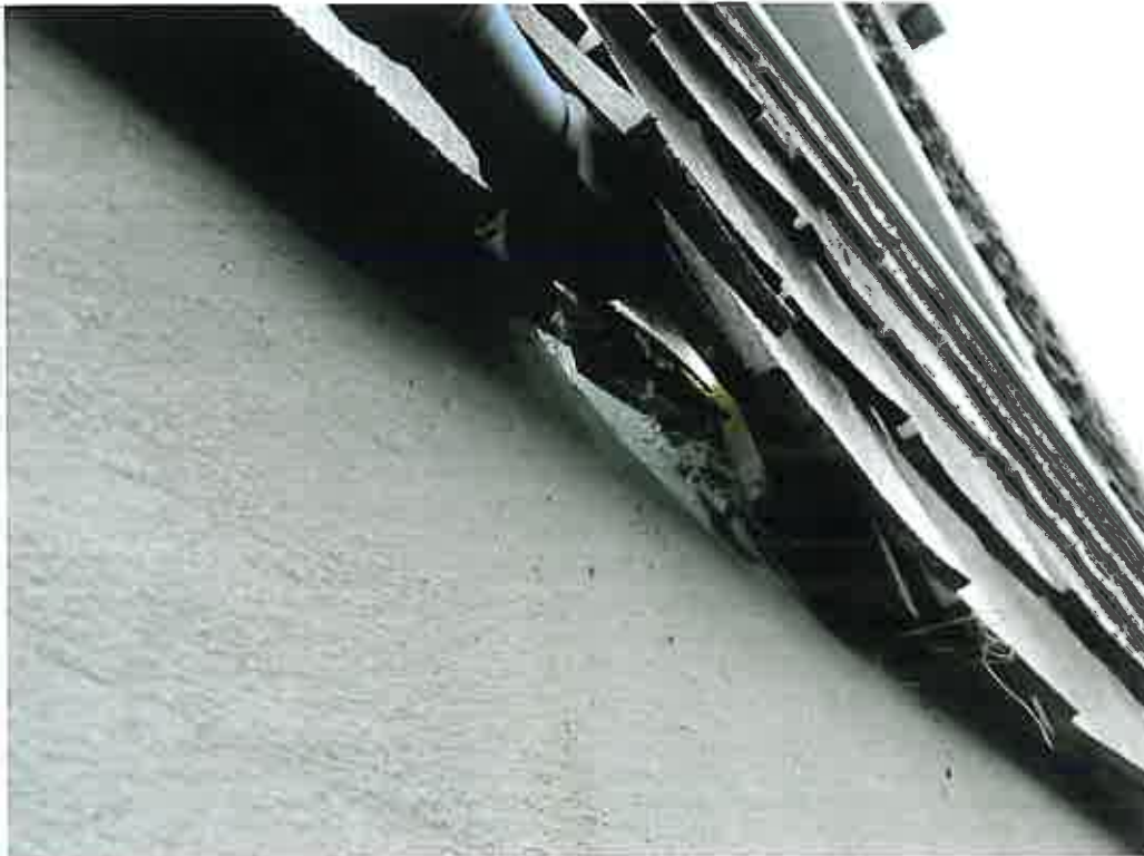
DETERIORATED OSB SHEATHING DIRECTLY BELOW A WINDOW (DIFFICULT TO MAKE OUT)
