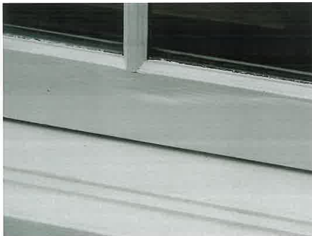
SEVERELY DETERIORATED WINDOW SASH
